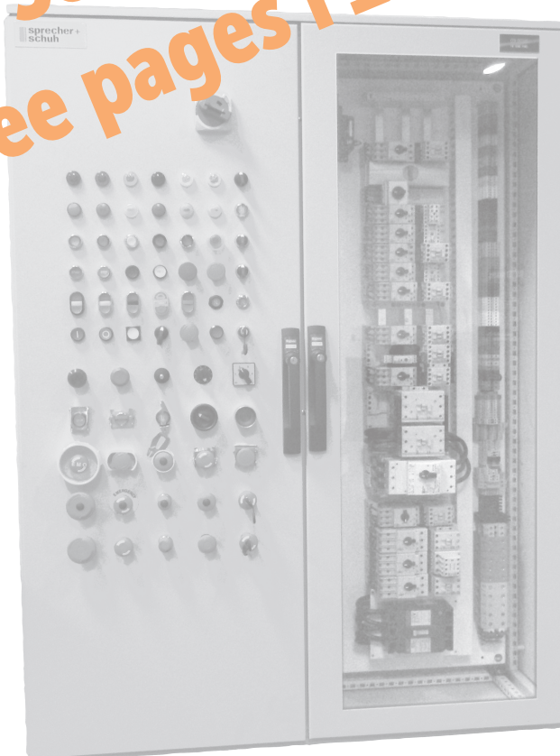
3-Phase 60mm Bus Bar System vertically arranged to maximize space
